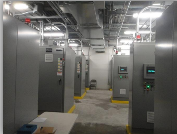
C88 Motor Control Room complete
